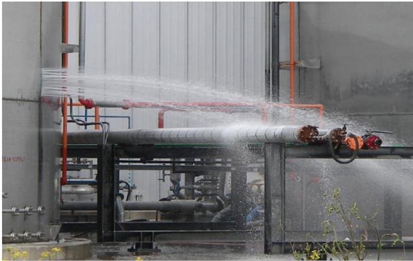
Acid leaking from side of storage tank at chemical facility.
